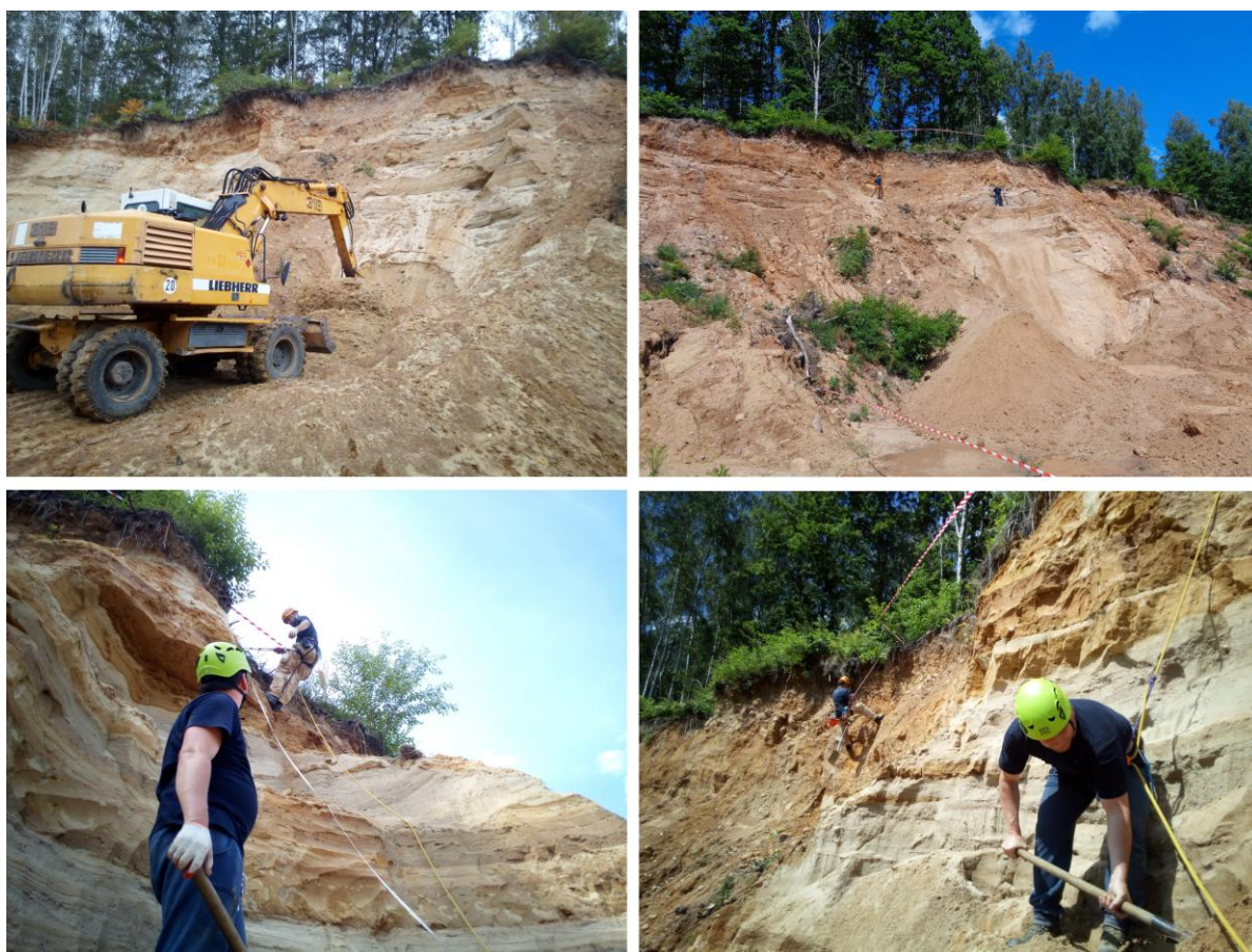
Figure 2 – Field works with the use of heavy equipment (excavators) and climbing harnesses while preparing an over 15-meter profile (photo P. Przepióra 2019)
