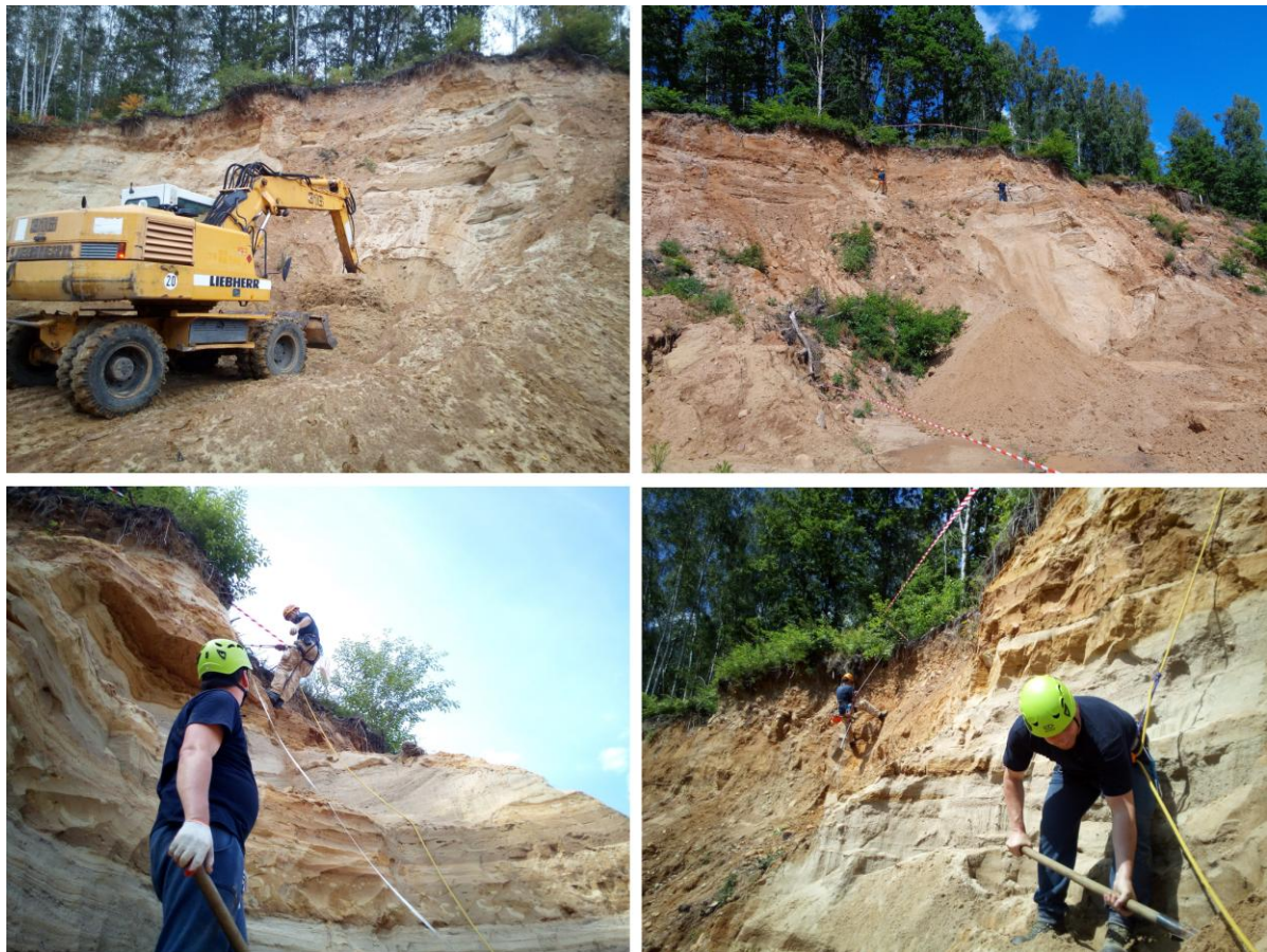
Figure 2 – Field works with the use of heavy equipment (excavators) and climbing harnesses while preparing an over 15-meter profile (photo P. Przepióra 2019)
